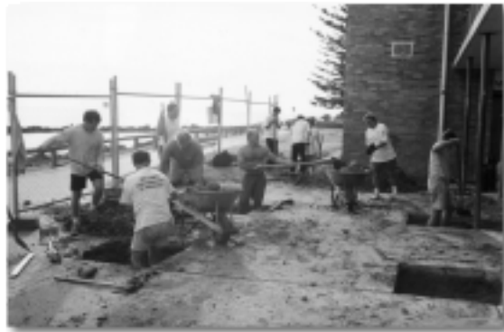
The new deck extension is underway and this is how it began
